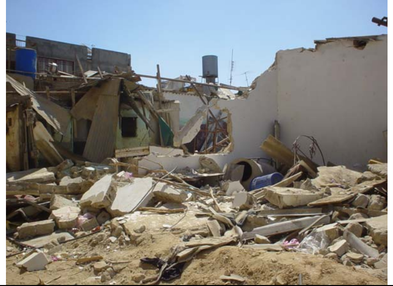
Photo 3: This is the home of Rasha's neighbors one house east of hers.
