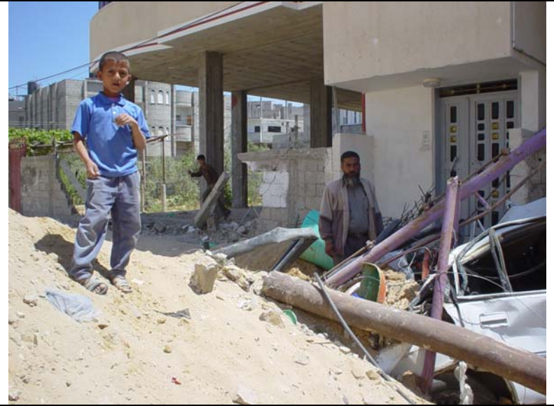
Photo 6: Damage to Palestine Women's Union Preschool in Rafah. Purple metal is from playground equipment.
