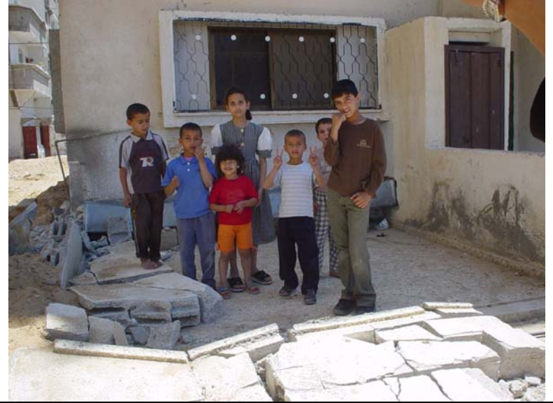
Photo 7: View of backyard of PWU Preschool. Boundary wall at the children's feet was knocked down by bulldozers.
